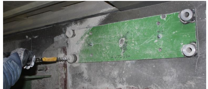
Drilling of the outer holes for further anchors installations. It was used a special metal jig to be ensured the verticality of the holes.
